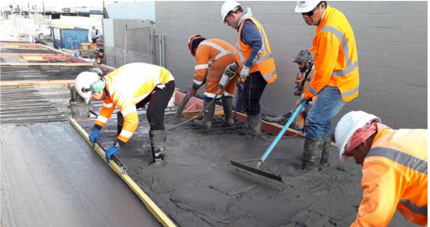
Works underway behind the New Lynn RSA on the corner of Hetana Street and Totara Avenue – undertaking the very first concrete pour as part of the Project in May 2020.
