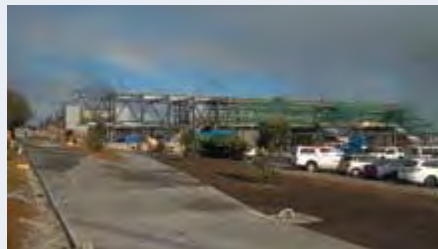
Steel trusswork for the concourse now largely complete. Scaffolding in place to enable installation of glazing.
