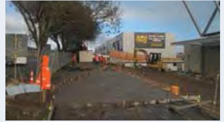
Formation of shared cycle path (with feature paving inserts defining local maunga (volcanic cones & peaks)).
