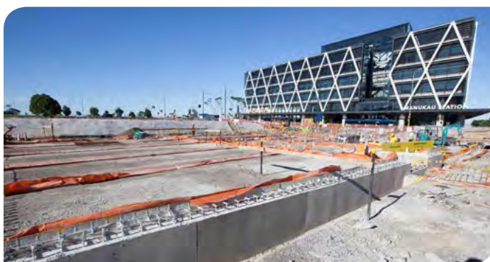
Concrete ground beams have been poured over conduits in a grid layout
