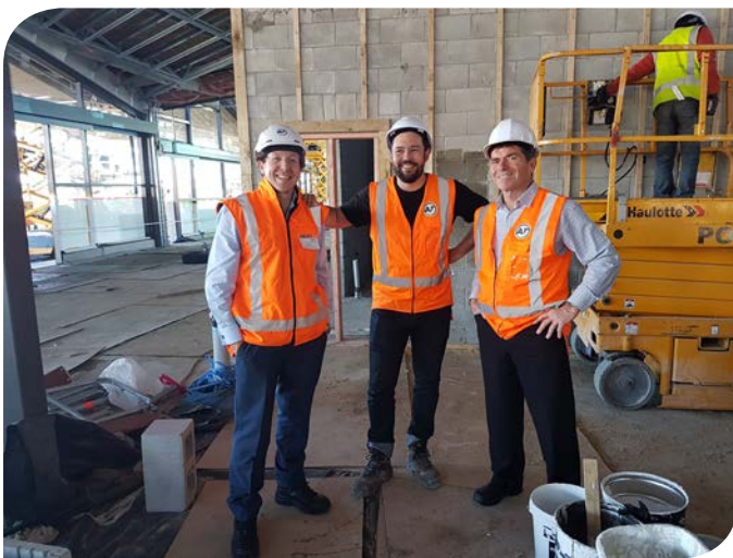
Auckland Transport's Mark Hitchcock, Scott Keene and Sean Corbett look happy with progress. AT has seven retail spaces available for lease in the bus station
