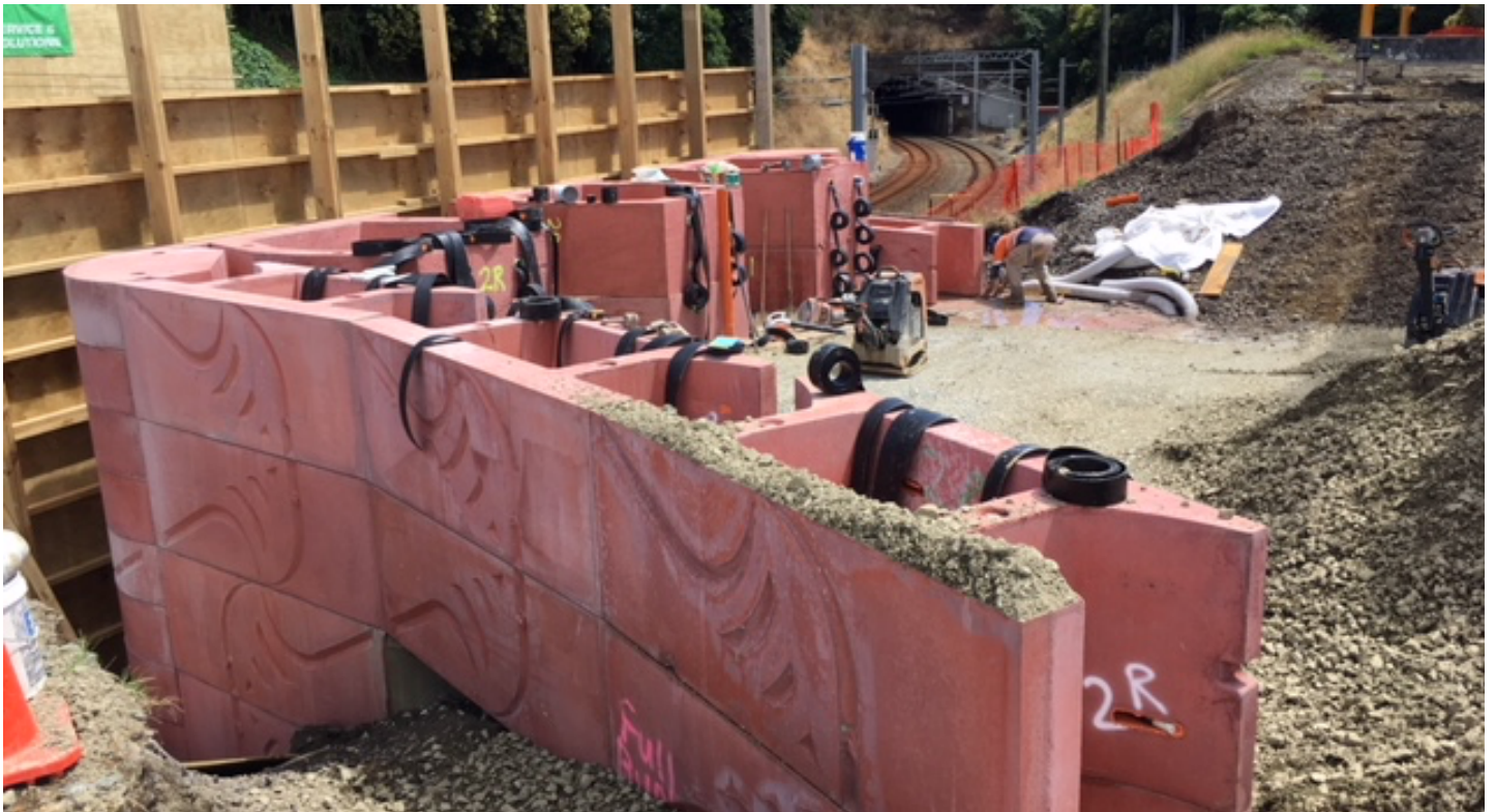
The East Abutment blocks are being placed in preparation for the bridge piling works to start
