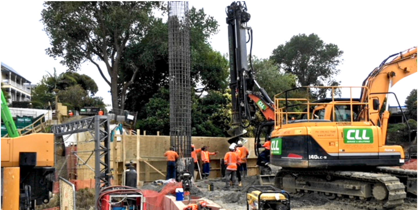
The Eastern Abutment bridge piles being constructed. In the centre, you can see the reinforcing cage being lowered into one of the pile holes. Immediately to the right (behind the white helmets), the piling rig and auger is working on one of the other piles. There are three piles of 1.2m diameter and 20m depth in each of the two bridge abutments.
