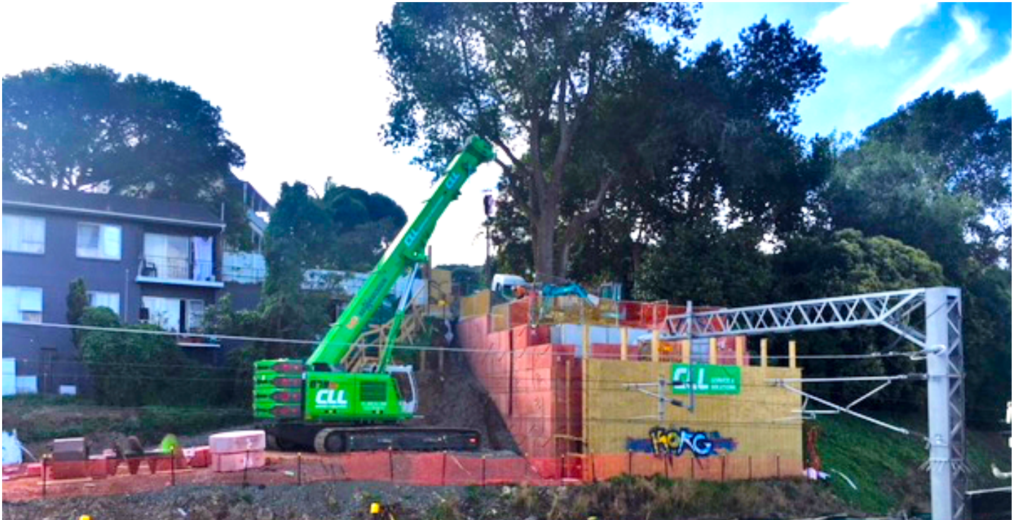
Good progress on the Western Abutment can be seen behind the hoarding. The blocks currently in place are generally about 1 layer below the finished height. You can see the temporary grey blocks to the left of the top of the gantry. These are being used to create a temporary level surface for the piling rig.
