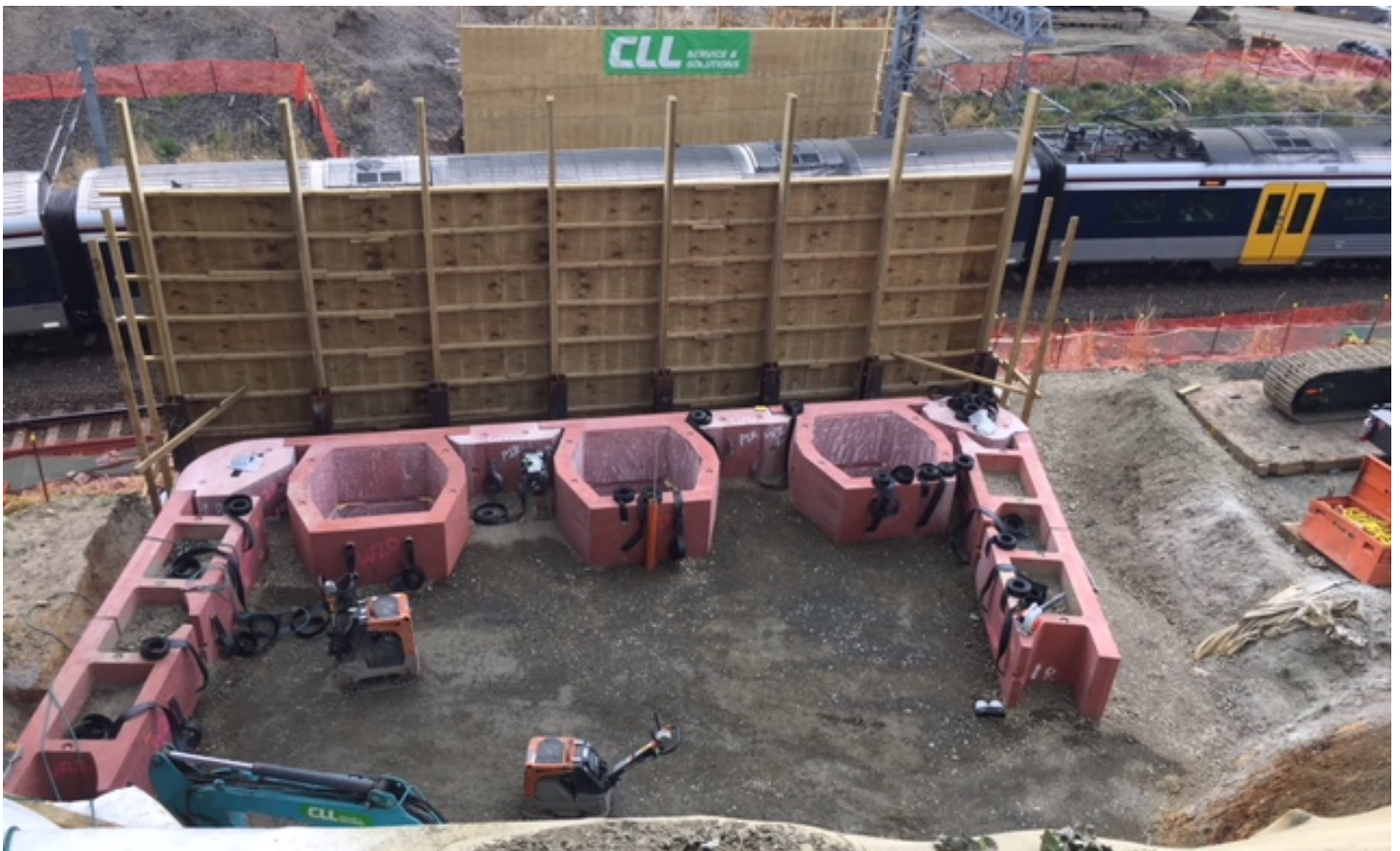
The West Abutment blocks and hardfill taking shape. Hoardings separate worksite from the rail tracks
