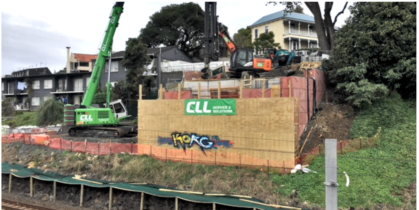
Piling work in progress on Western Abutment (centre). Green crawler crane on left for removal this week
