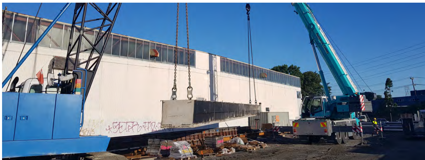
Bridge Beams being lifted out of the mould at the precast yard in Otara.
