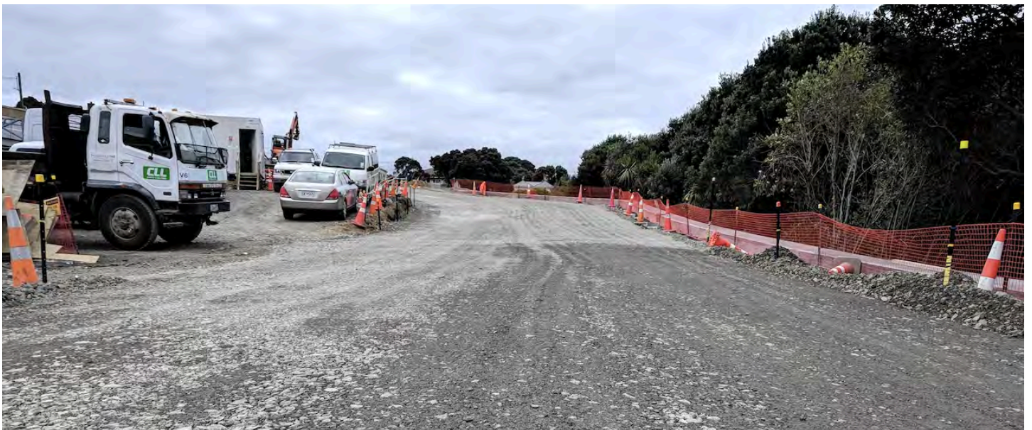
Subgrade in place on the new section of Laxon Terrace ready for the subbase
