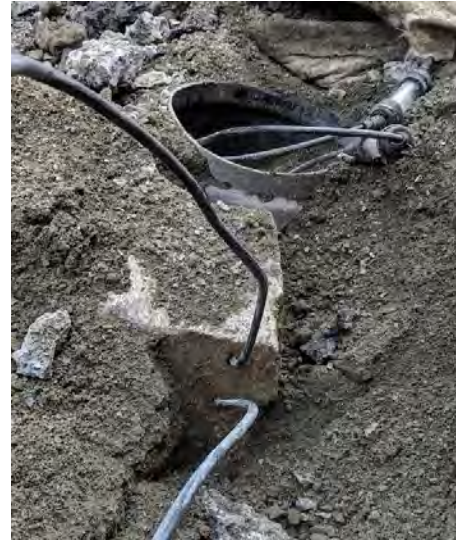
Cable with no protective ducting
