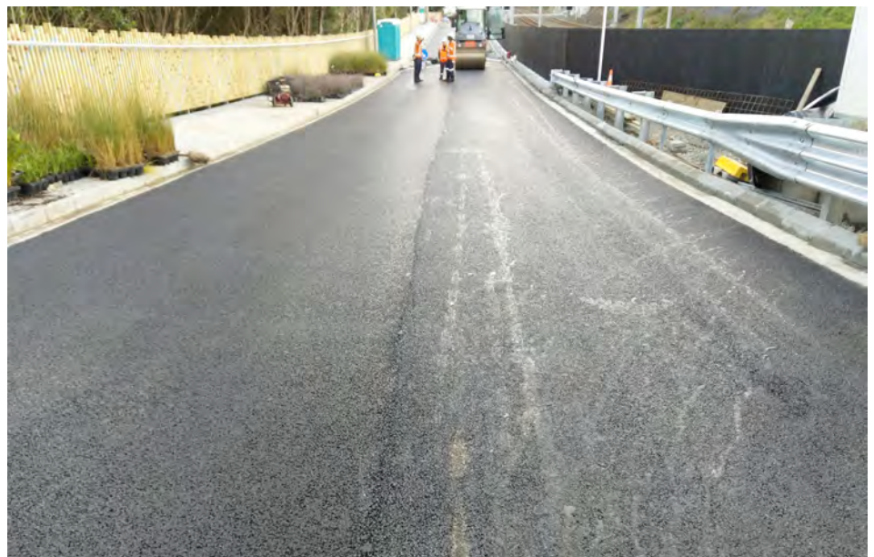
Laxon Terrace sealing complete. Mana Whenua fencing alongside footpath. Wooden fence alongside rail tracks on right painted black.
