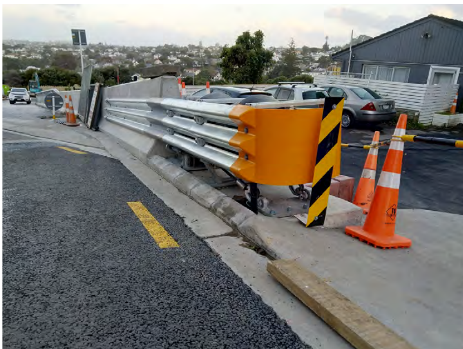
Crash cushion outside 9 Cowie Street
