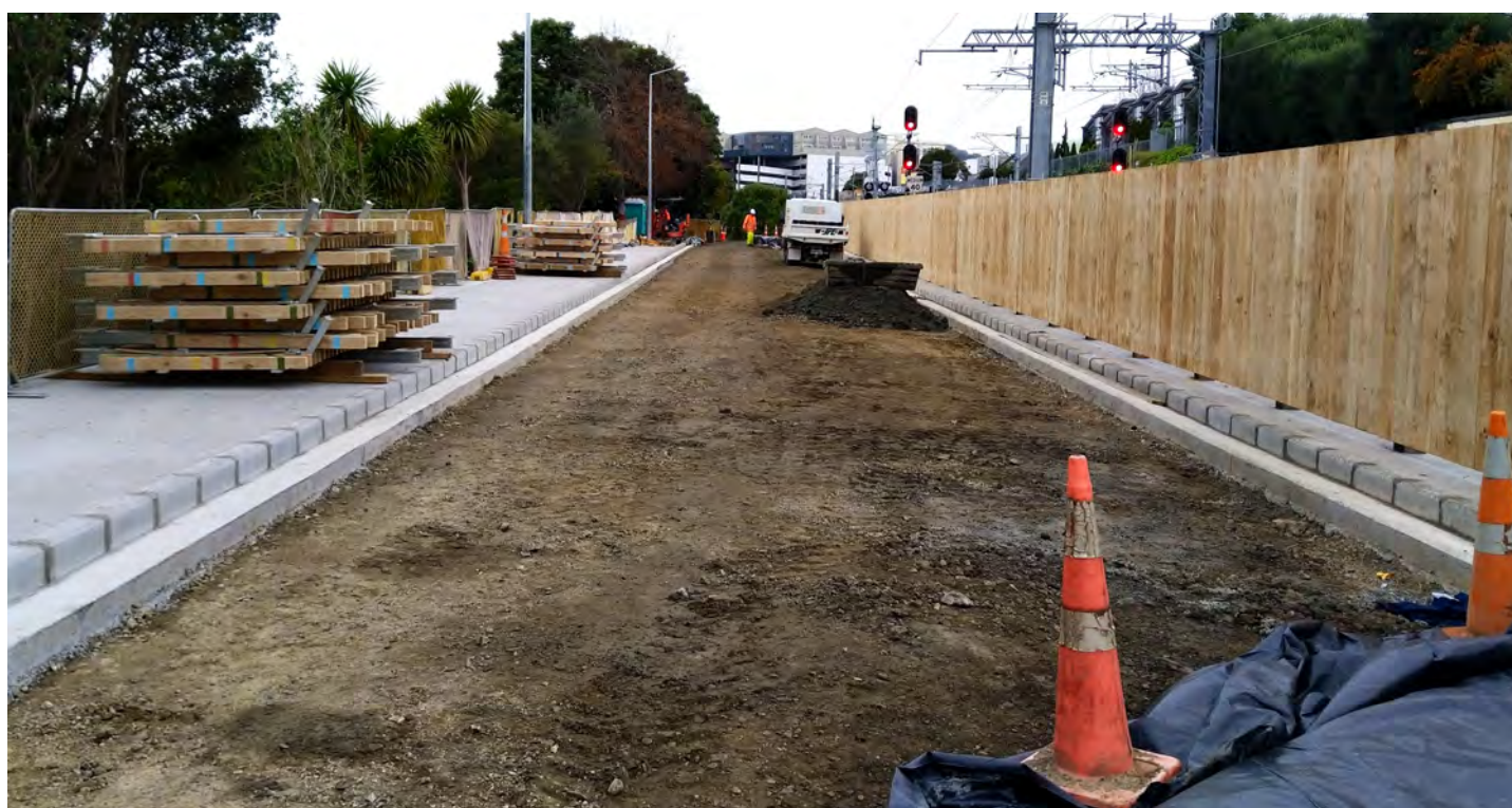
Looking south along new section of Laxon terrace with new separation fence on the right
