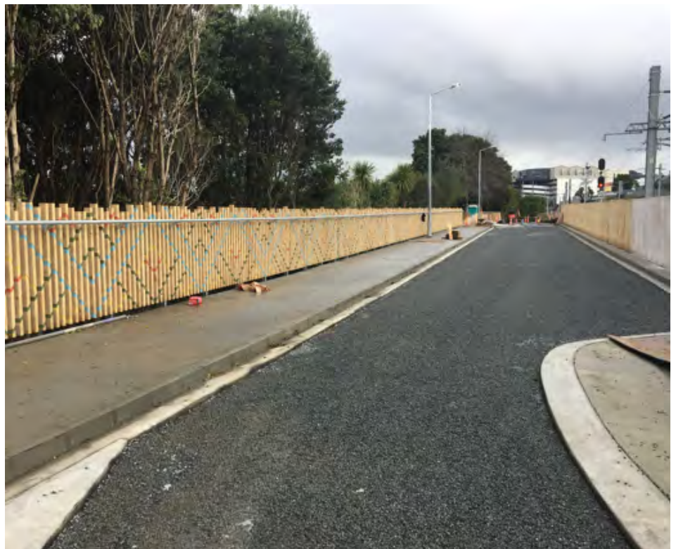
Mana Whenua fencing alongside footpath. Undercoating (white) being applied to wooden fence alongside rail tracks on right
