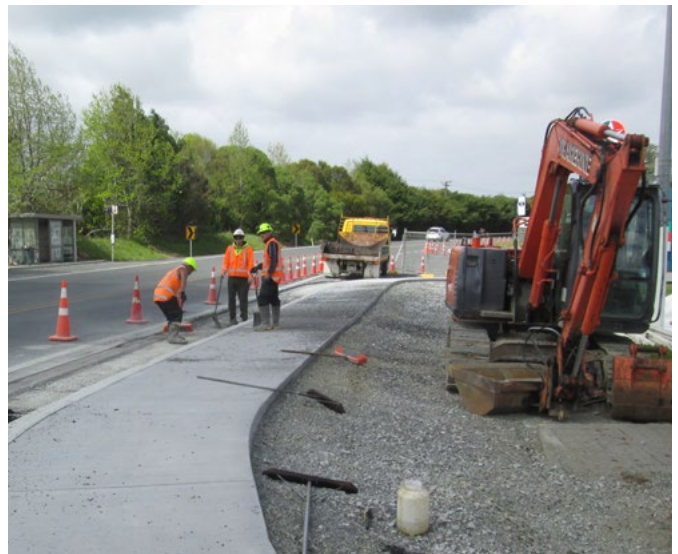
Extending the footpath to remove the left turn lane at the Kahikatea Flat Road intersection
