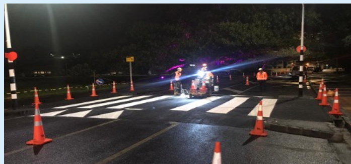
The finishing touches being put on the new raised pedestrian table on Tamaki Drive, which was finished on Tuesday night.
