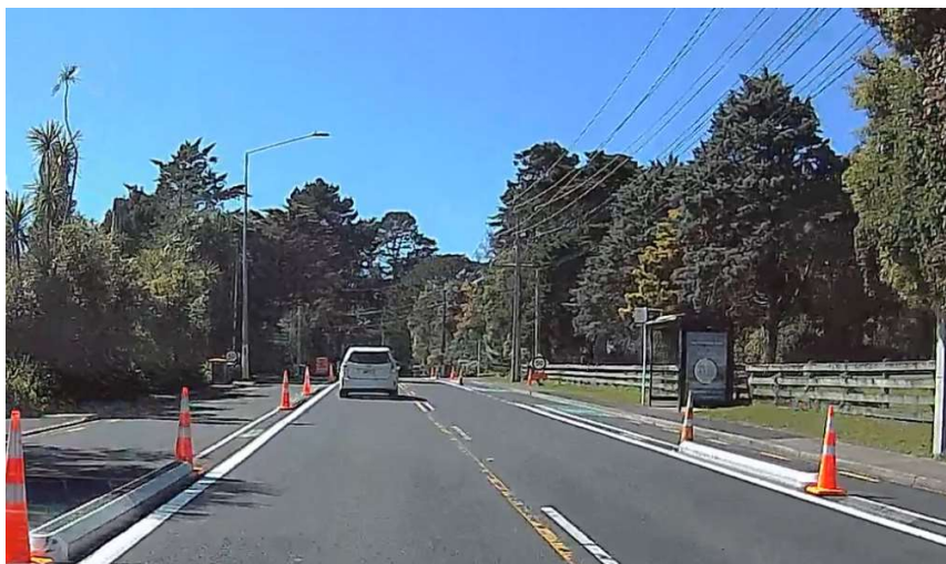
Figure 5. Faded line markings and narrow lane widths on northern section of Upper Harbour Drive.
