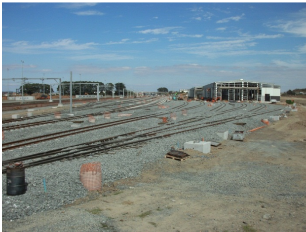
Fig 2: Trackwork and overhead line is well advanced and construction of the perimeter fence has commenced
