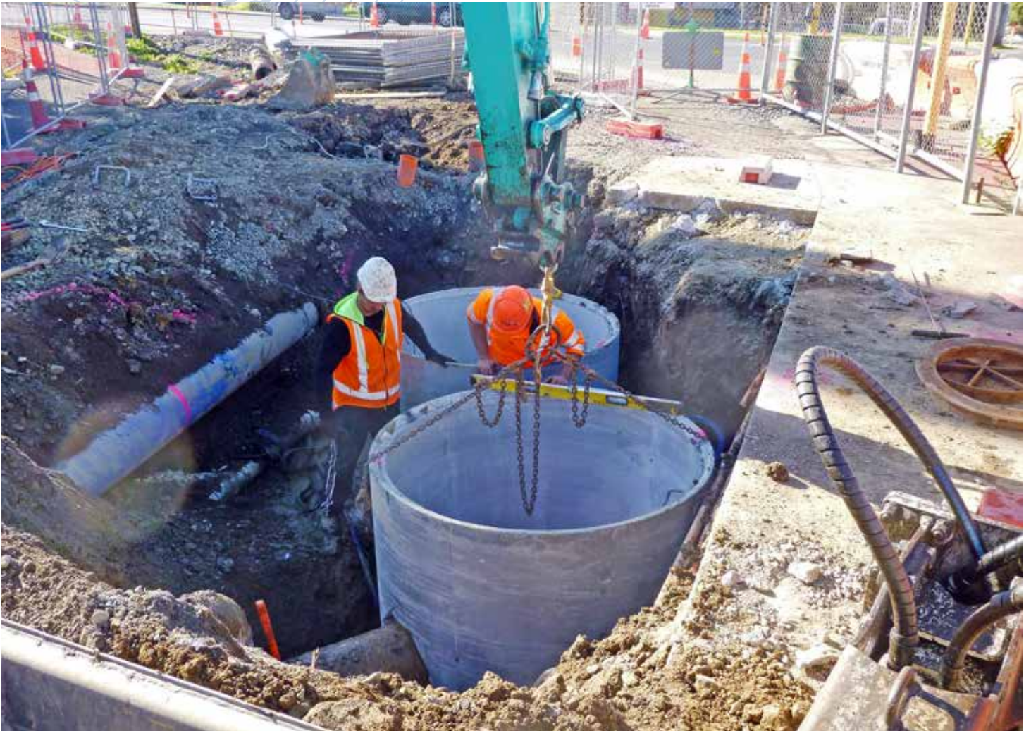
Above: Installing new stormwater and sanitary sewer manholes on the corner of Forrest Hill and Wairau Roads
