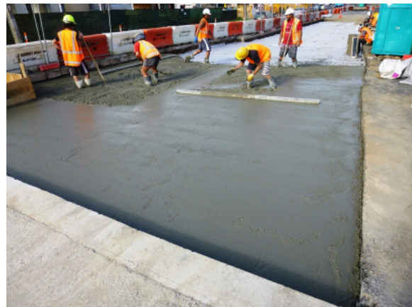
Placing new concrete on Wairau Road on the approach to the bridge
