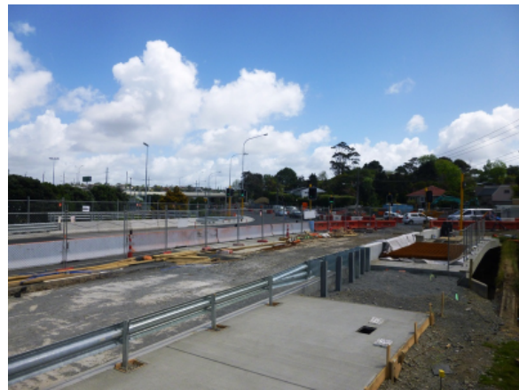
View of the new bridge including the guardrail and footpath on Wairau Road
