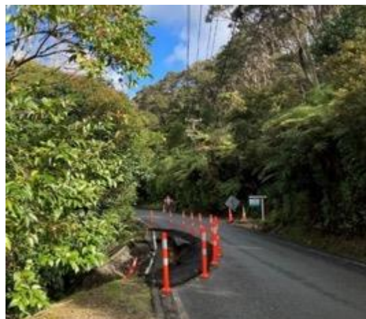
Slip site on Kellys Road Oratia, road will be fully closed during works.
