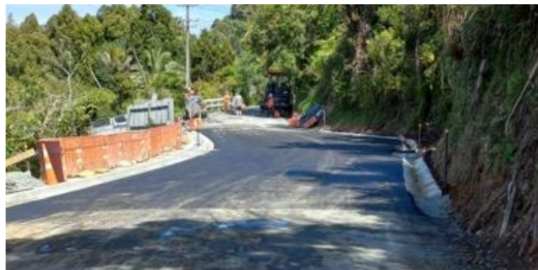
Retaining wall, near completion and road seal going on Forest Hill Road, 25 September 2024.
