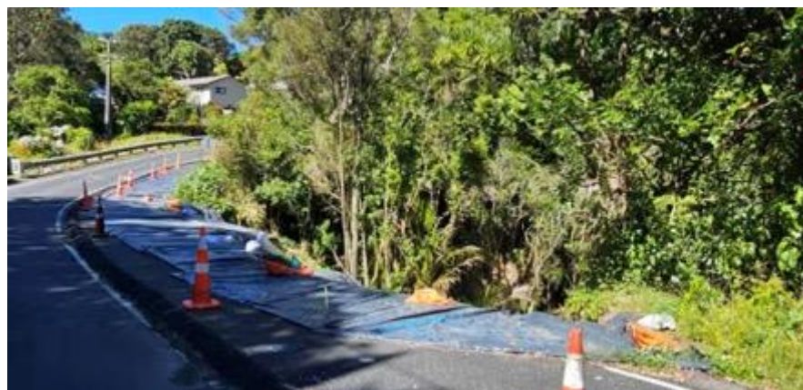
Woodlands Park Road Slip Site
