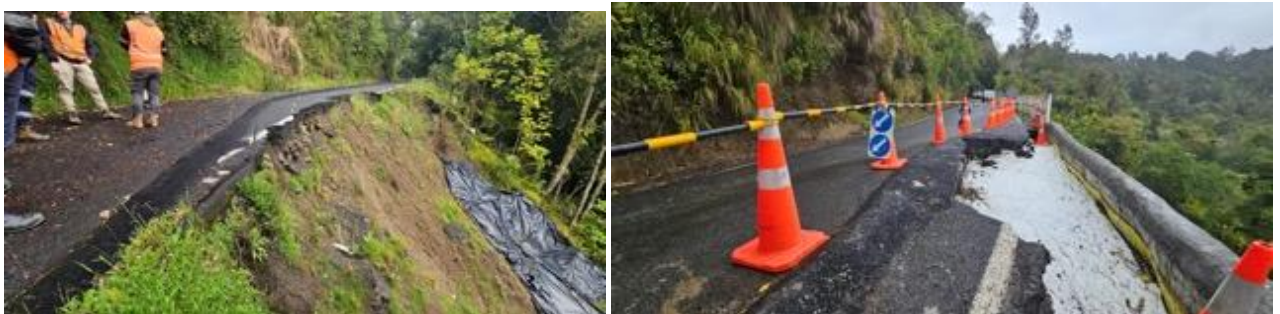
Work on Mountain Road – images shows the narrow nature of Mountain Road, works underway on sites.
