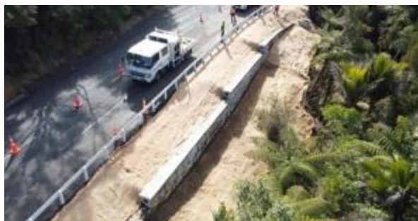
Block retaining wall completed, seeding and matting has been done and we expect to see the grass growing through soon.
