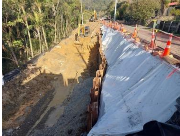
Slip repairs underway on Te Henga Road, temporary sheet pile wall installed central to the picture.
