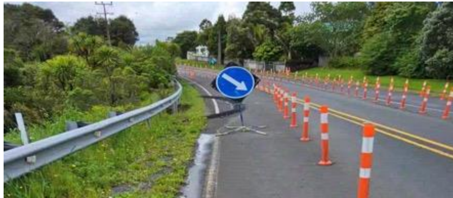
West Coast Road, Oratia slip site.
