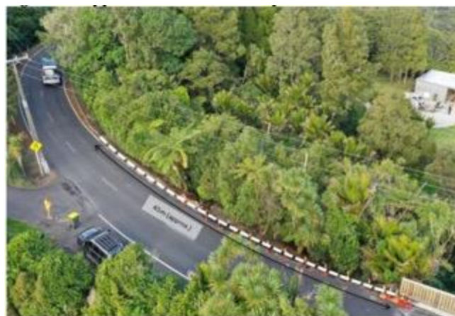
Wairere Road slip site 349 Wairere Road
