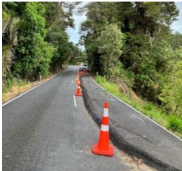
Site ready to start works once the large site at RP8.25 is complete.
