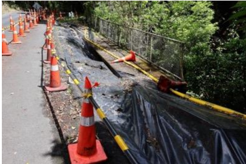
Konini Road Slip Site
