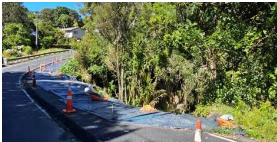
Woodlands Park Road Slip Site
