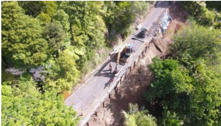
Site RP1.387 Mountain Road – image shows the sheet piles installed and preparation for drilling.
