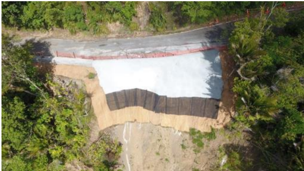
Work at RP1.664 Mountain Road – images show the work underway during November.
