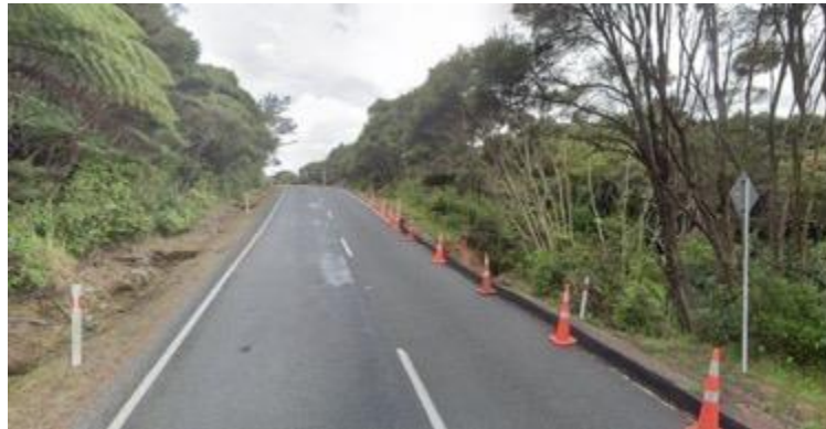
Slip located approx. 100m past Cornwallis Road intersection.
