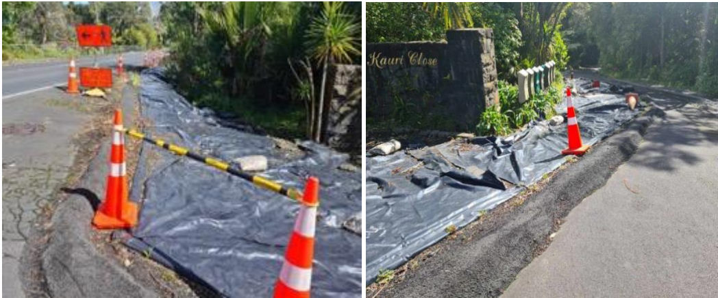
Slip located near at 81 Huia Road.
