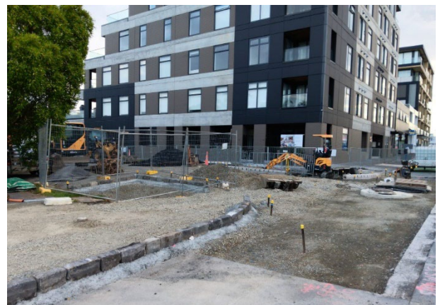
Base layers of the side road entry treatment at Northland St. Can you see the new tree pit on the corner of Northland St?
