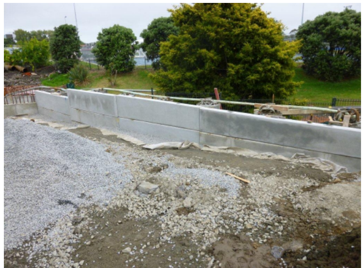
Retaining wall being constructed on the Albany side of the new Wairau Creek Bridge.
