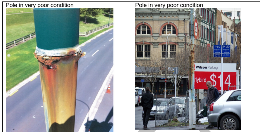
Figure A 7: Examples of street lights requiring replacement
