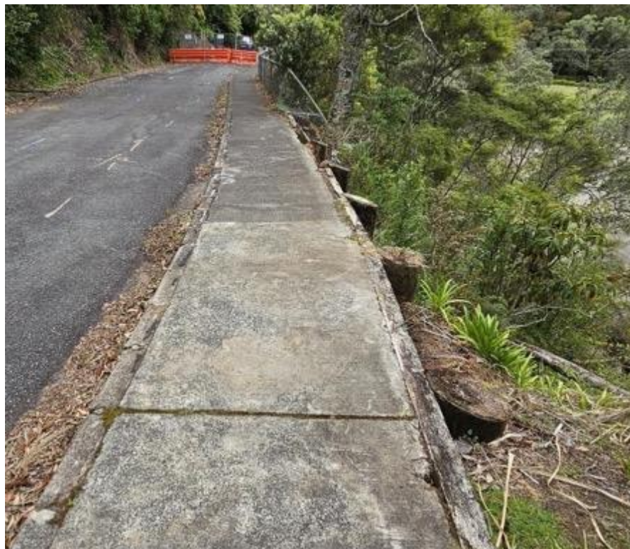
Large Slip on the corner of Paturoa Road, previous retaining wall has failed and fallen towards the beach.
