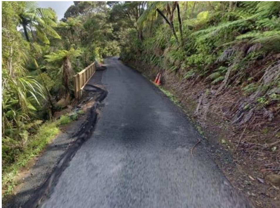
Slip site RP2.5 Lone Kauri Road, works started 15 January 2025. The handrail in the photo is above a retaining wall built prior to the cyclone. The retaining wall will be extended either side of this location.
