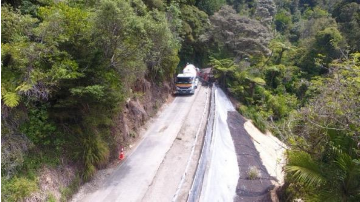
Site RP1.387 Mountain Road – image shows work on the kerb and channels.
