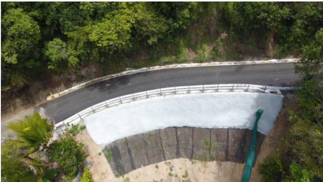
Work on Mountain Road – image shows the pavement completed at RP1.468 site
