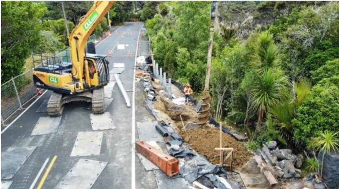
Slip located at 81 Huia Road, work underway installing piles for the retaining wall in early January 2025
