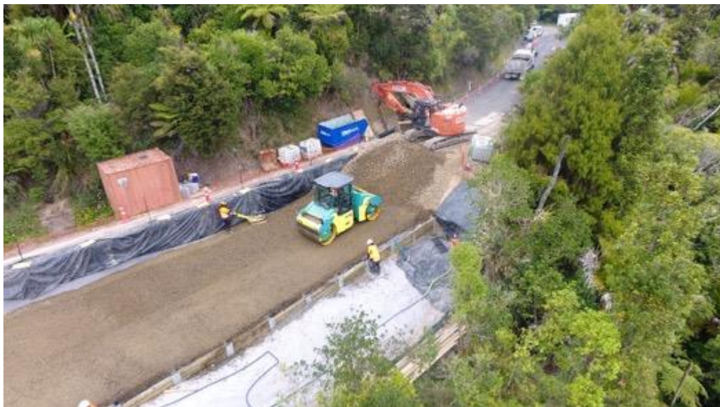
Scenic Drive RP6.73 site – the permanent retaining wall and works commencing behind the wall to rebuild the road.
