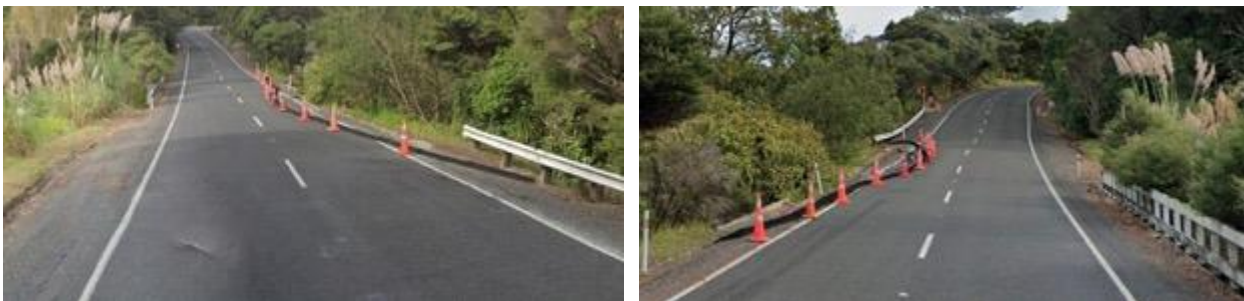
Site RP12.55, currently there are retaining walls on each side of the road, large upstream catchment and existing stream.
