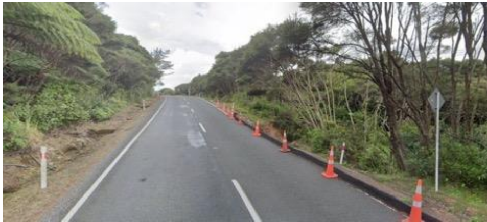
Slip located approx. 100m past Cornwallis Road intersection.
