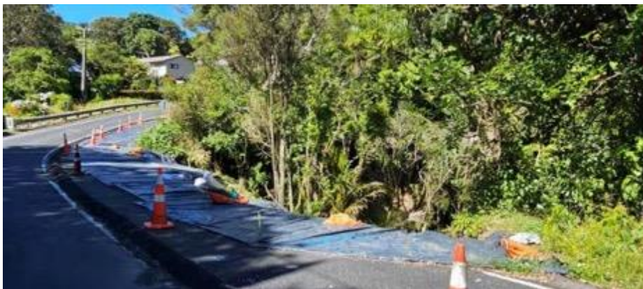
Woodlands Park Road Slip Site
