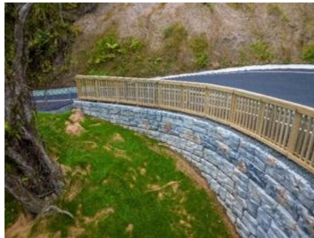
Slip site RPO.582 Karekare Road, completed installation of the rediblock wall and guardrail.
