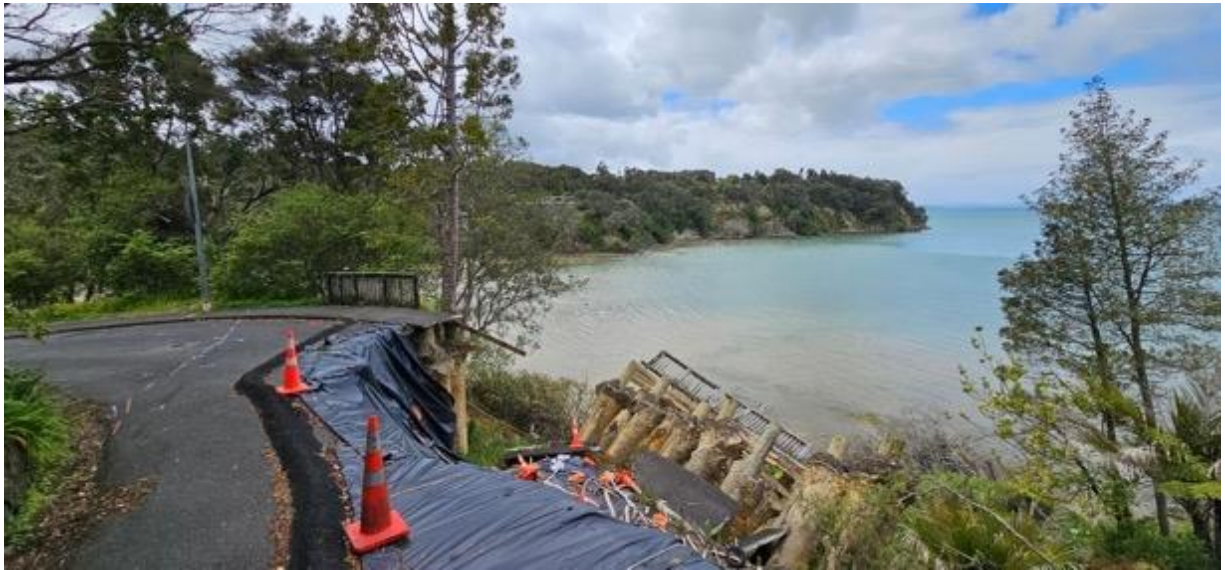
Large Slip on the corner of Paturoa Road, previous retaining wall has failed and slipped towards the beach.
