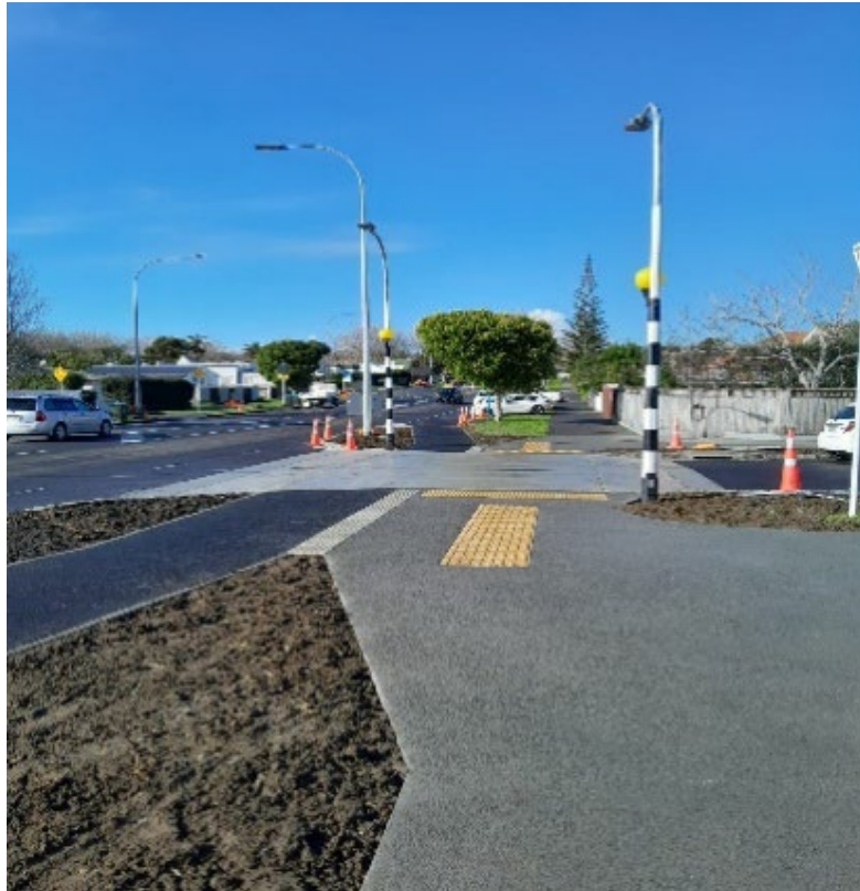
Image of Westmere Crescent and new raised crossing – line marking still to be completed.
