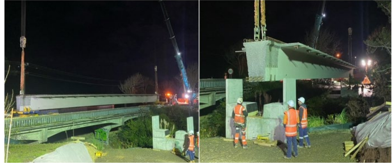
RODNEY TARGETTED RATE – Rail overbridge installed for footpath project, SH1 / Rodney St, Wellsford
