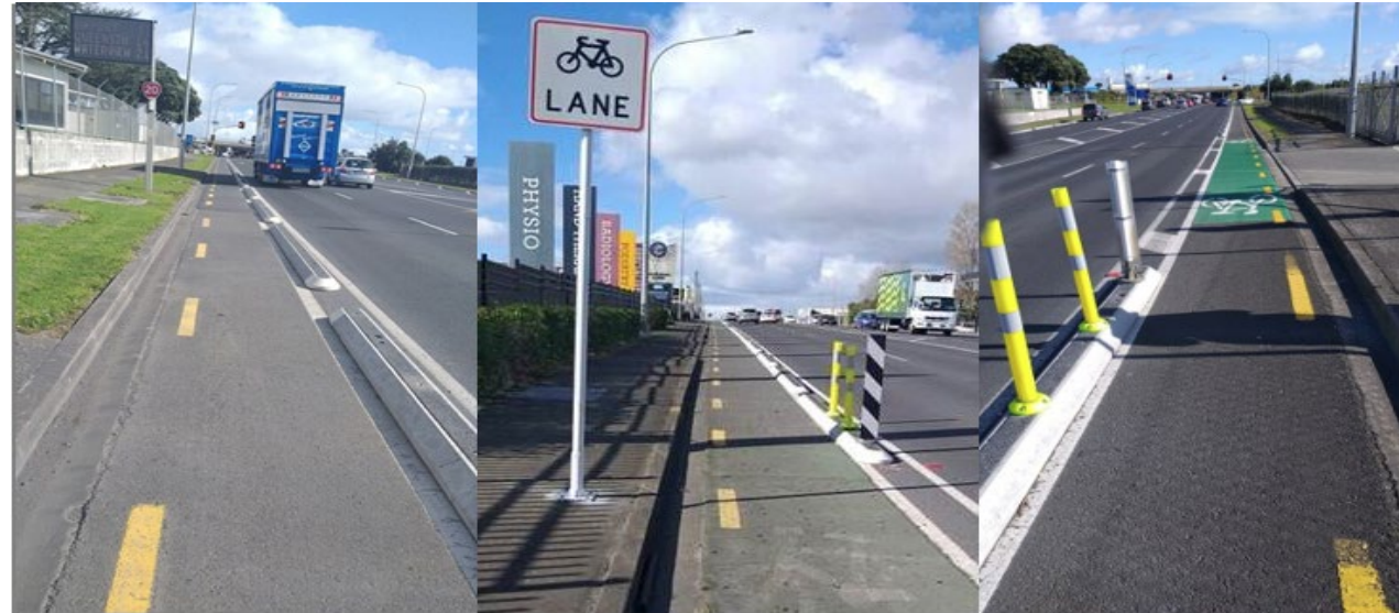
CYCLING - Cavendish Drive, Manukau – installed new low profile concrete separators and improvements to existing cycleway
