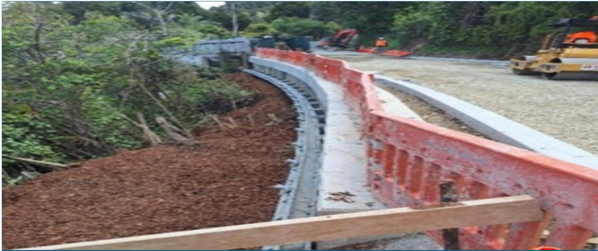
Forest Hill Road, Waiatarua open for traffic in September and currently works are in progress
